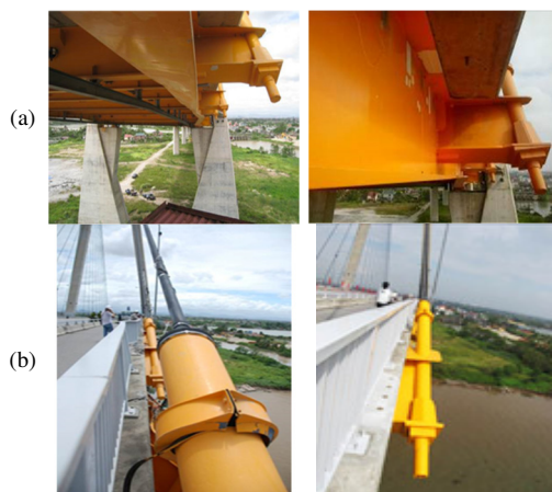
Fig. 4. General arrangement of Binh Bridge and the location of the bridge damage in 2010. (a) a. In 2010, when damaged, (b) in 2012, after repairs.
