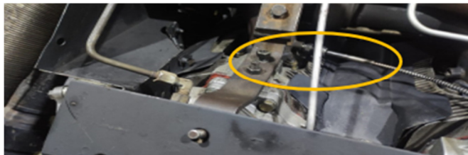
Fig. 4. Temperature sensors installation position.
