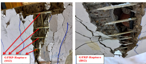
Fig. 8. Rupture in GFRP-bars in specimens SS2 & BS2.
