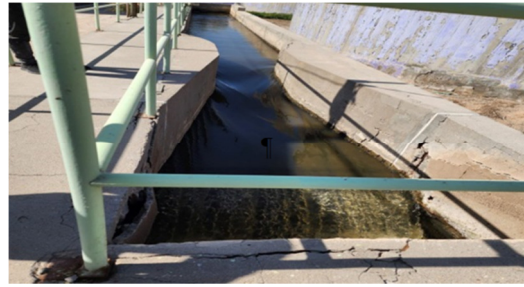
Fig. 2. Untreated wastewater before it is disposal into the river.
