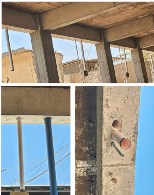
Fig. 1. Various service pipes passing through RC beams in commercial buildings.
