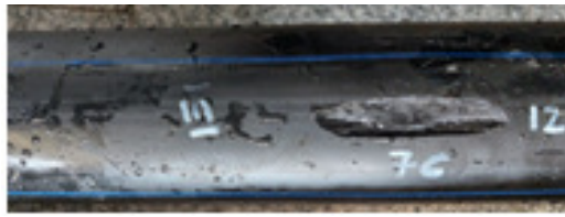
Fig. 16. Splitting in Pipe III.
