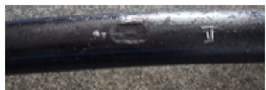
Fig. 15. Cracking in Pipe II.
