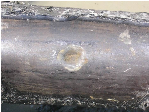
Fig. 1. Defects as local deformations detected on the pipelines.
