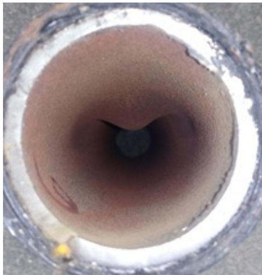
Fig. 6. Fracture of the pipe material.
