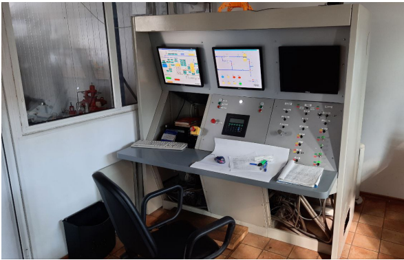
Fig. 2. Command and control console of the compressors test bench.
