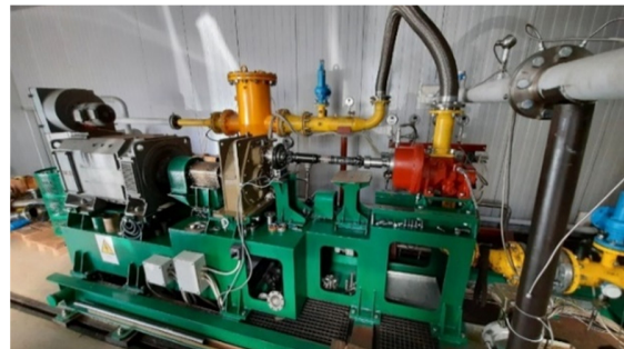
Fig. 1. Compressor skid within the test bed.
