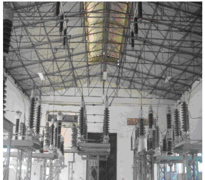
Figure 1. View of the 66kV enclosed air substation at Linoperamata
