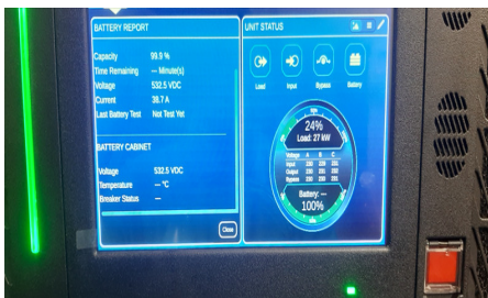
Fig. 11. Battery report from the UPS.
