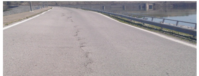
Fig. 10. The displacement on the earth dam's crest.
