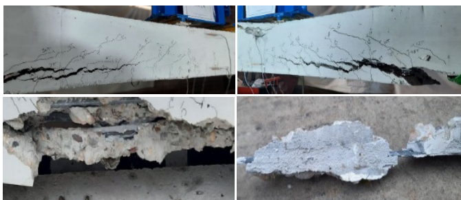
Fig. 9. Concrete cover separation and debonding of CFRP laminates.
