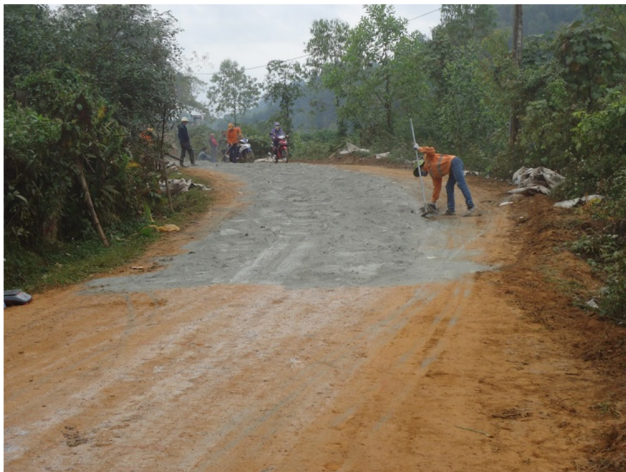
Fig. 1. Cement and/or fly ash placement on the road before mixing with local soil underneath
