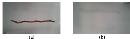
Fig. 3. (a) Horizontal crack in house C, (b) repaired
