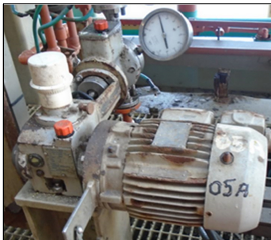
Fig. 3. Hypochlorite injection dosing pump
