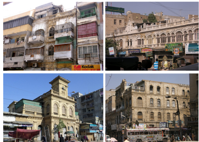
Fig. 3. Images showing encroachments and various forms of vandalism on historic buildings.
