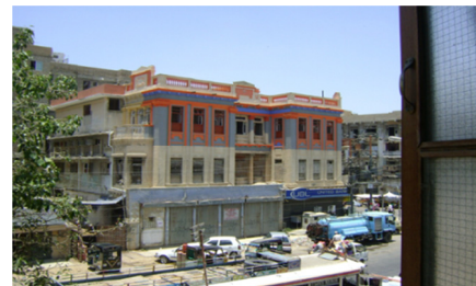
Fig. 4. Image showing unwanted repairs in form of application of paints as surface decoration over stone facade
