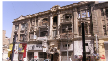
Fig. 1. Krishna Mansion in Saddar Bazaar (highly deteriorated)
